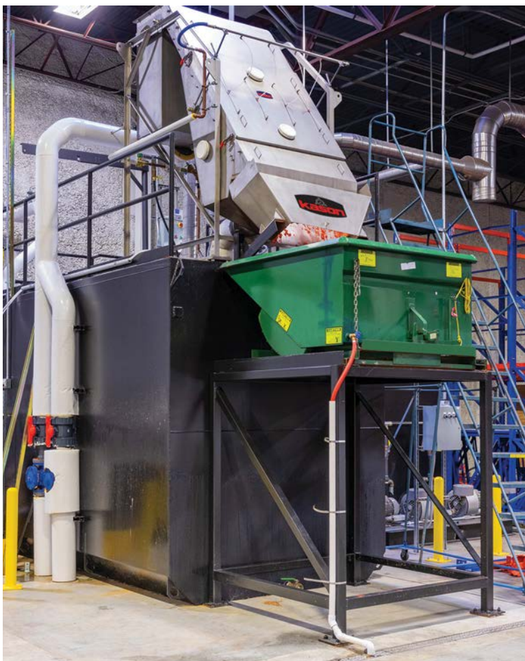
Cross-Flo Sieve Removes Solids from 106,000 l Per Day of TGD Cuts' Wastewater before it Enters the Municipal Wastewater System.
