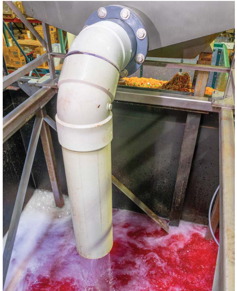
Screened Wastewater is Pumped to the Municipal Wastewater Plant in Compliance with Accepted Levels of Total Suspended Solids.
